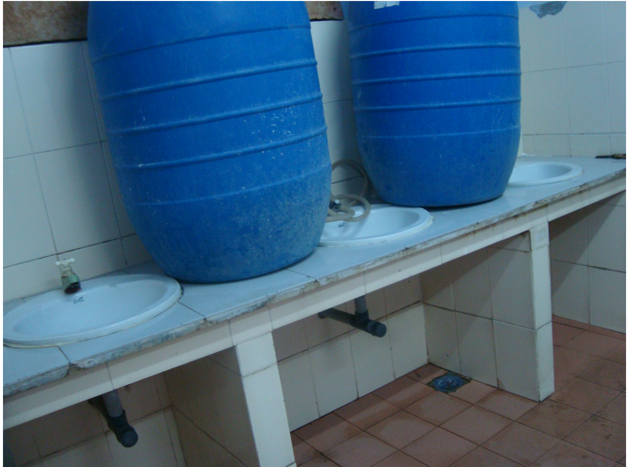
Figure 6: Broken sinks in the patient's toilet
